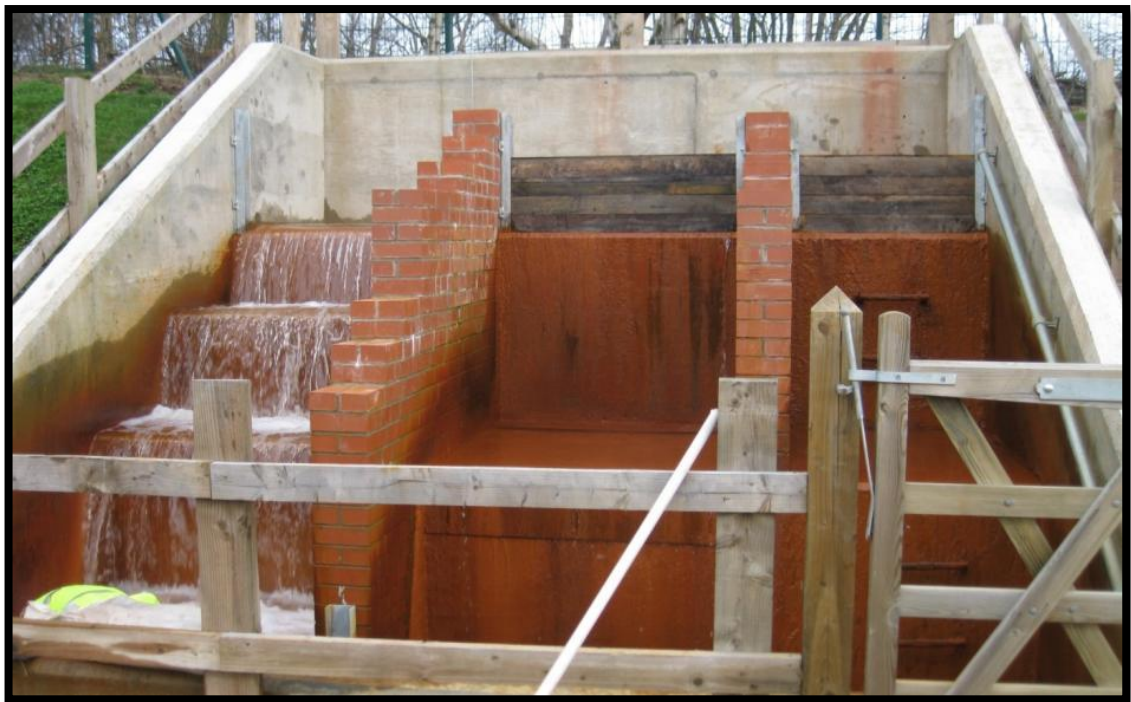
Figure 4-4 Aeration cascades at Strafford (full view)
