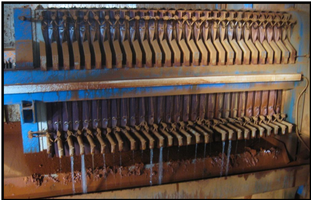
Figure 2-13 Filter press for sludge dewatering at Dawdon
